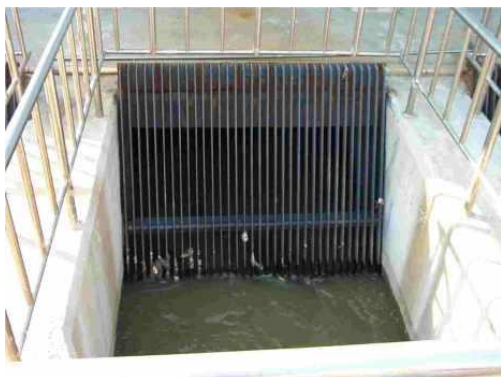
Manually cleaned bar screen
